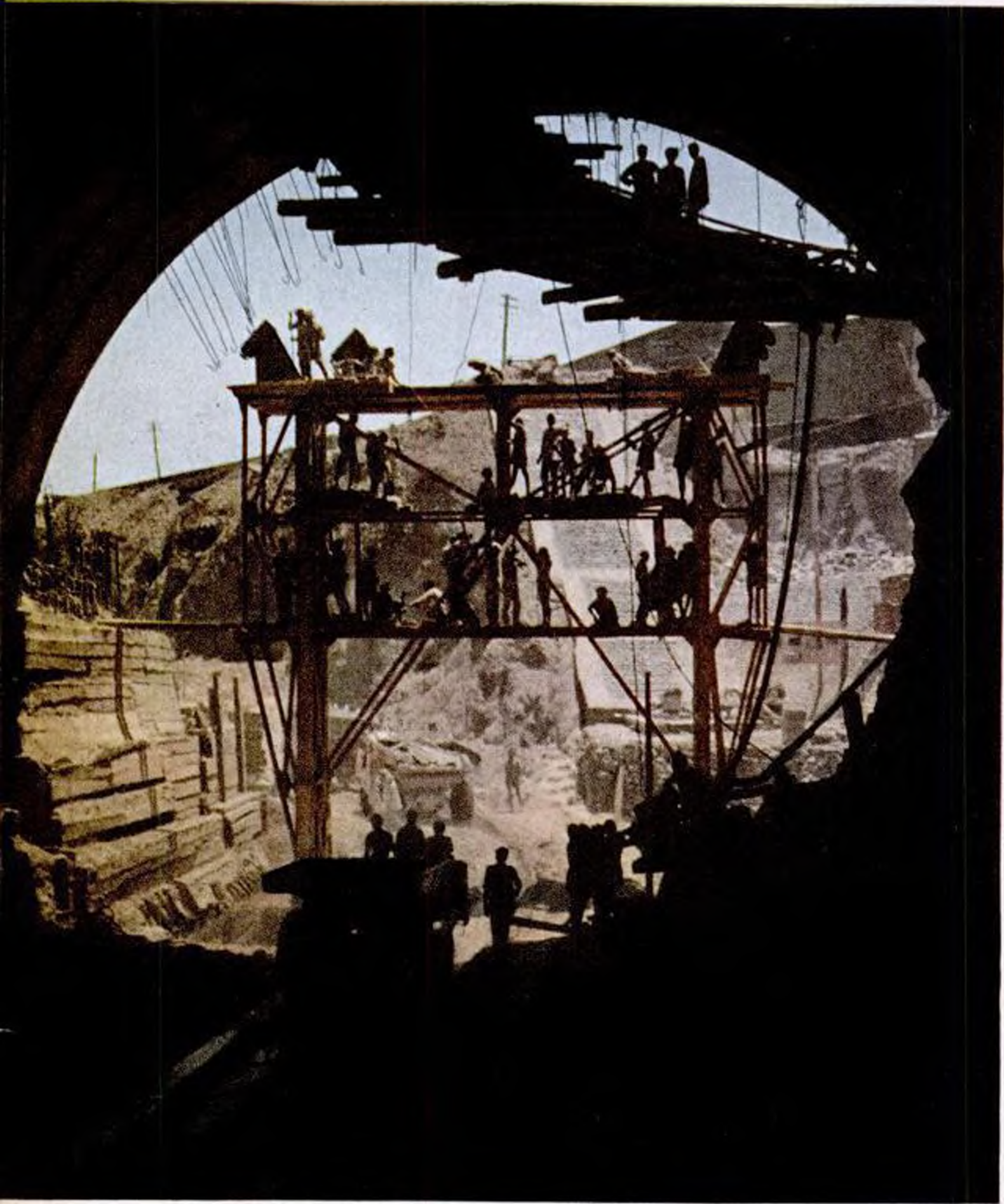
OPENING A TUNNEL. earth movers clear rock from the 60-foot Bhakra Dam diversion bore, while workmen put up scaffold to apply tunnel's concrete liner.
